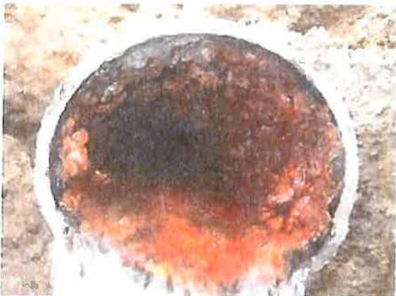
Tuberculated Water Line
